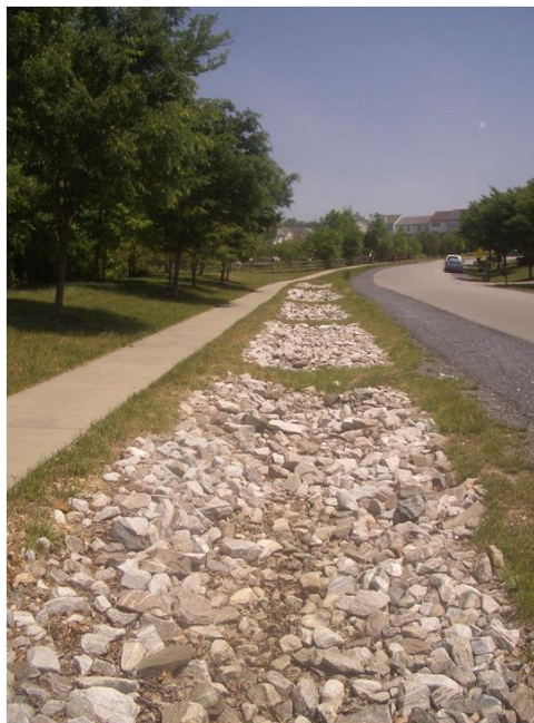
Example of infiltration trenches with stones in urban area
